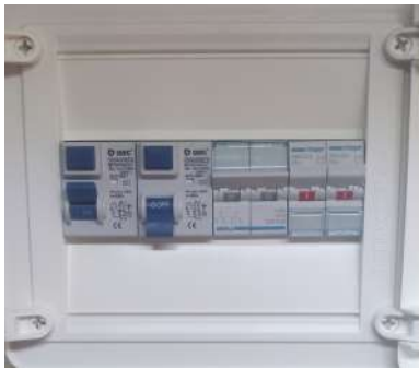
(a) Electric board panel
