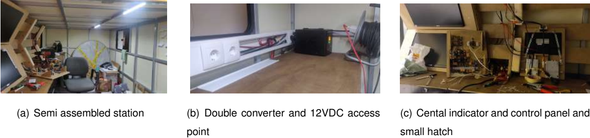
Figure 6.4: Wiring of some of the 230VAC and 12VDC grids
